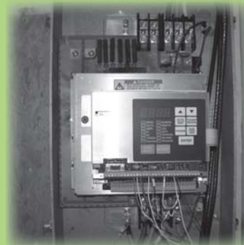
Complex control panel of new disperser unit requires special wiring and operation.
