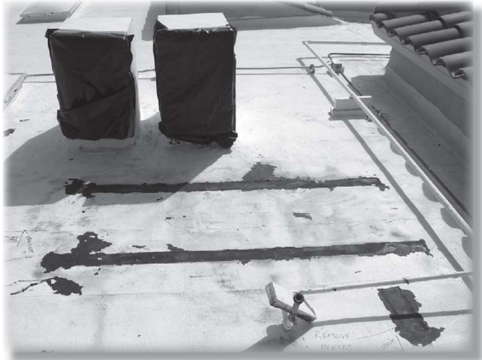
The above photo shows how the roof has deteriorated under the removed HVAC unit.
