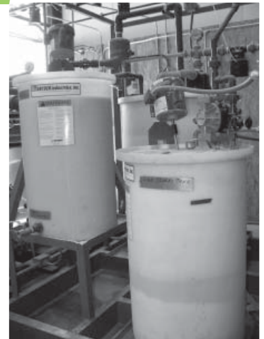
Water travels through the treatment processes
