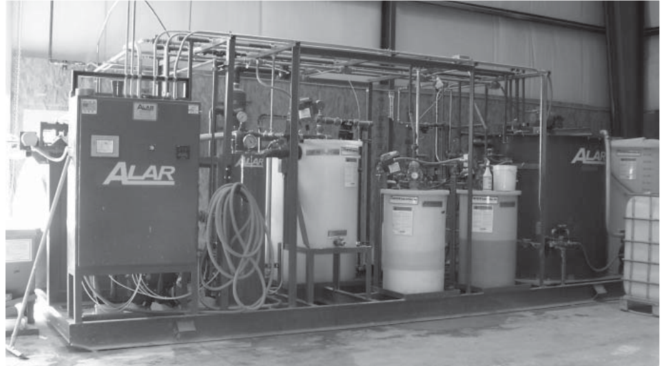
The ALAR Flex-O-Star water reclaimant is an expansive automated system.
