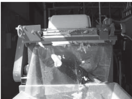
Solids accumulate on the revolving drum above, the variable-speed knife removes the solids from the drum's surface, then deposits in a dumpster.
