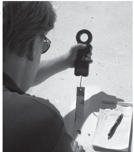
Jerry Rockwell uses a scale to perform a pull test on the roof to determine coating adhesion.
