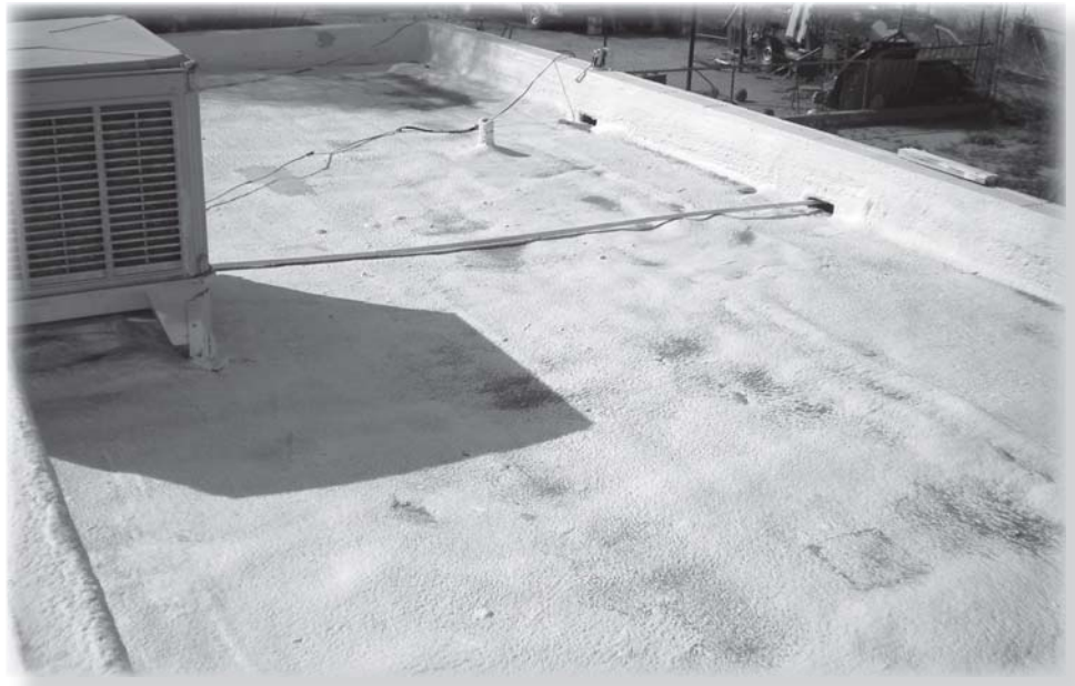
The worn spots on this coated foam roof could have been prevented with better maintenance. [Photo by Jonathon Montgomery]
